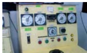
INDUCE VOLTAGE TEST SET
