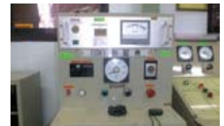
AC VOLTAGE WITHSTAND TEST EQUIP.
